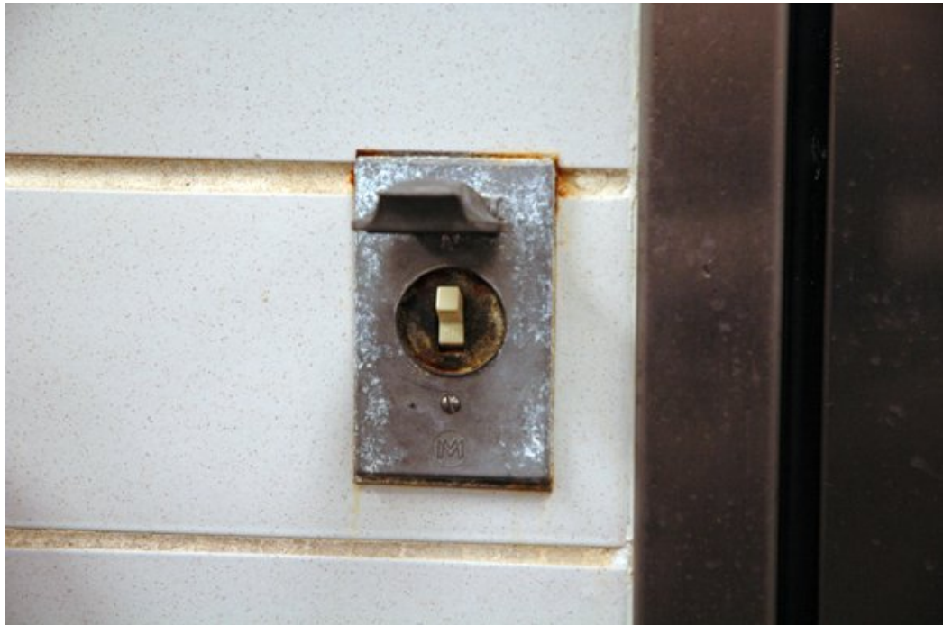
A light switch with residue build-up and grime. The switch could be contaminated with Lm by employees' hands during operation, and may not be cleaned during sanitation. When the light is turned on the next day, the hands could be re-contaminated.
