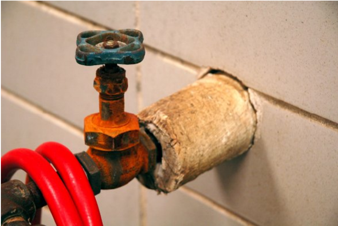
A rusty water spigot with a dirty, cracked insulated pipe. Lm could spread to the hose and be sprayed in the establishment.
