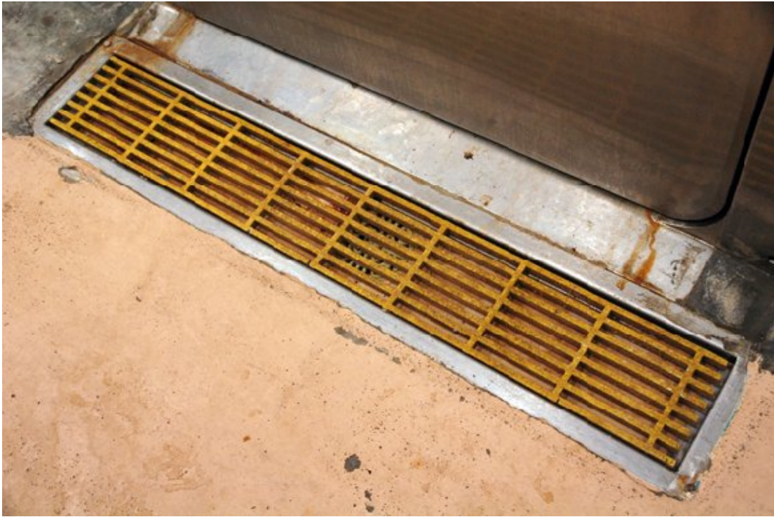
A drain at the entrance of a cooler doorway. The drain could become contaminated with Lm , and when employees step on the drain to enter the cooler, the Lm can spread into the cooler.
